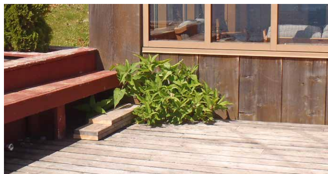
Knotweed is able to grow through decks and building foundations as this photo showing Himalayan knotweed demonstrates.
